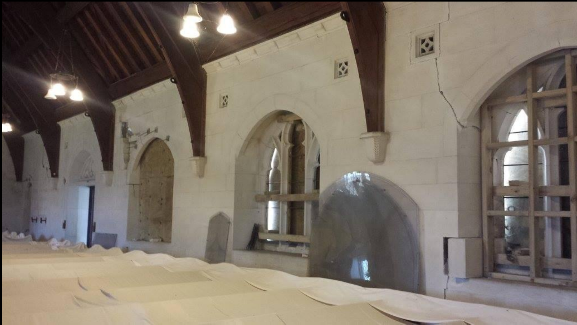
The damaged north wall of the nave at St Barnabas with windows removed for safe keeping.
