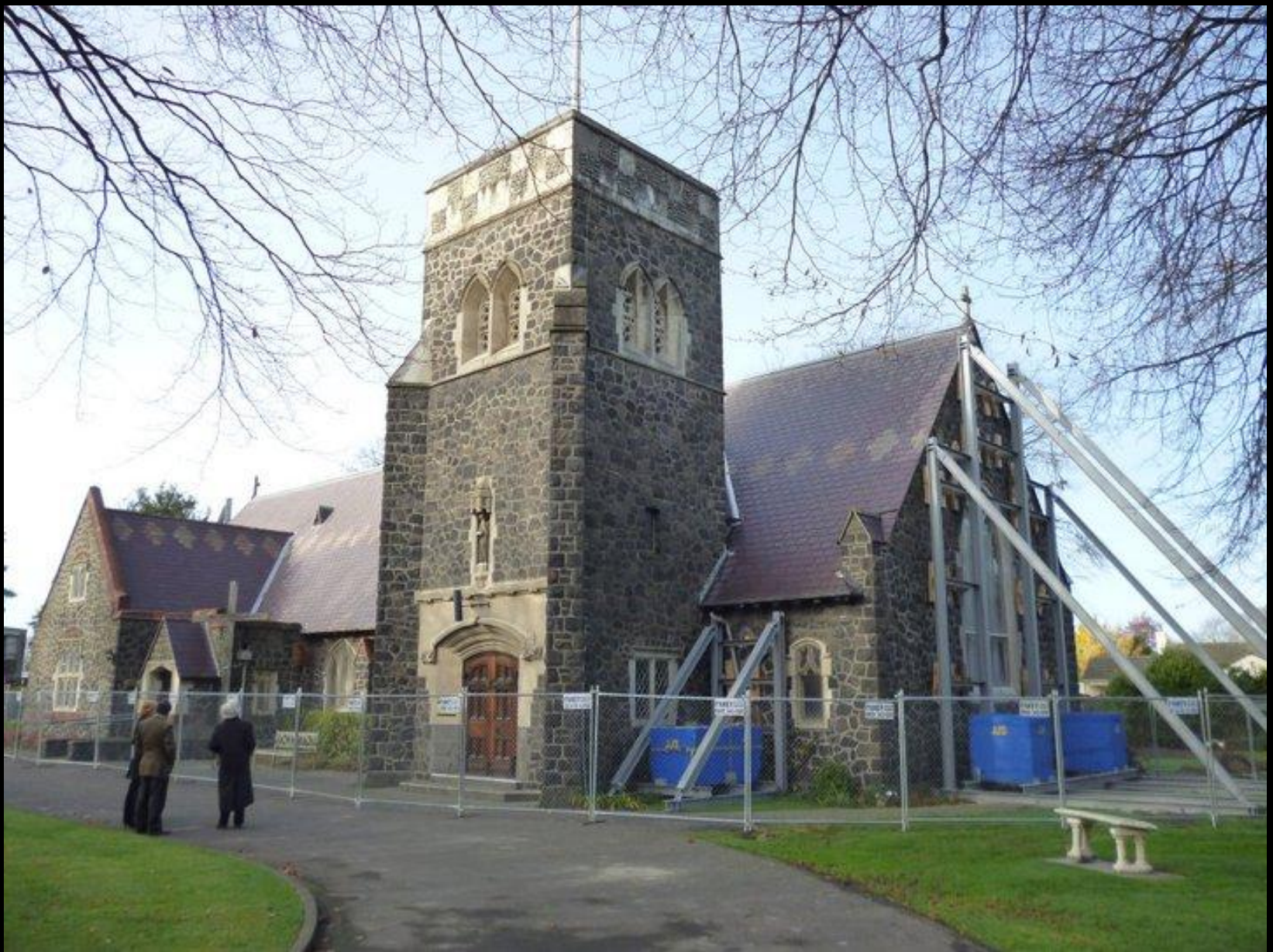
Still standing almost four months after the 22 February 2011 Quake, but there is extensive structural movement and cracking.
